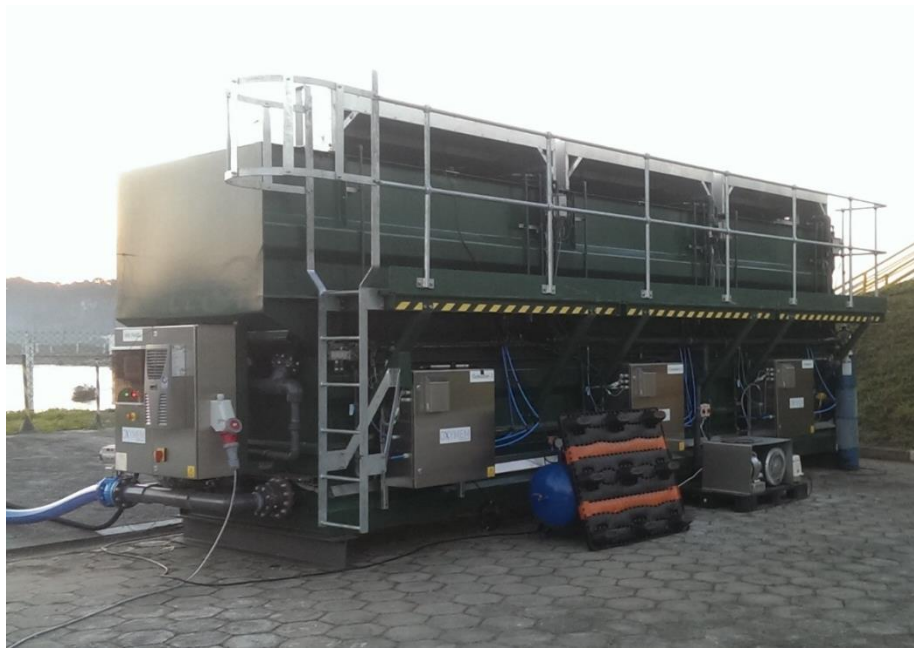
Figure 2: OxyMem MABR installed in Aruja Brazil
